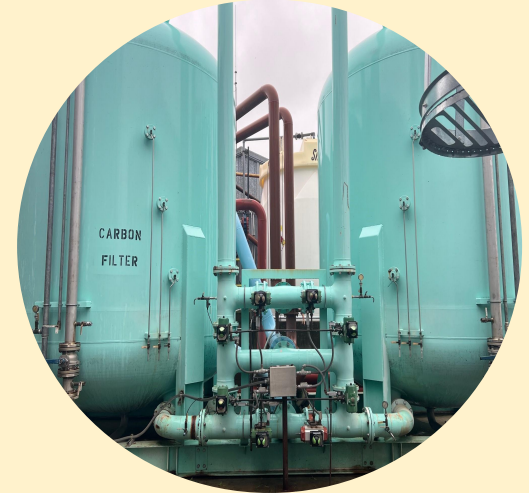
New Carbon Contactor at the Plant
