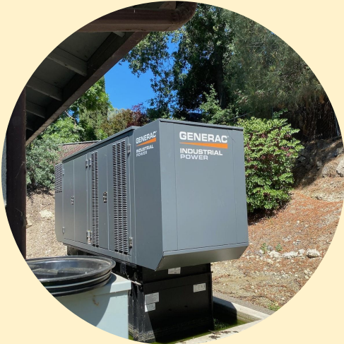
New Generator System
